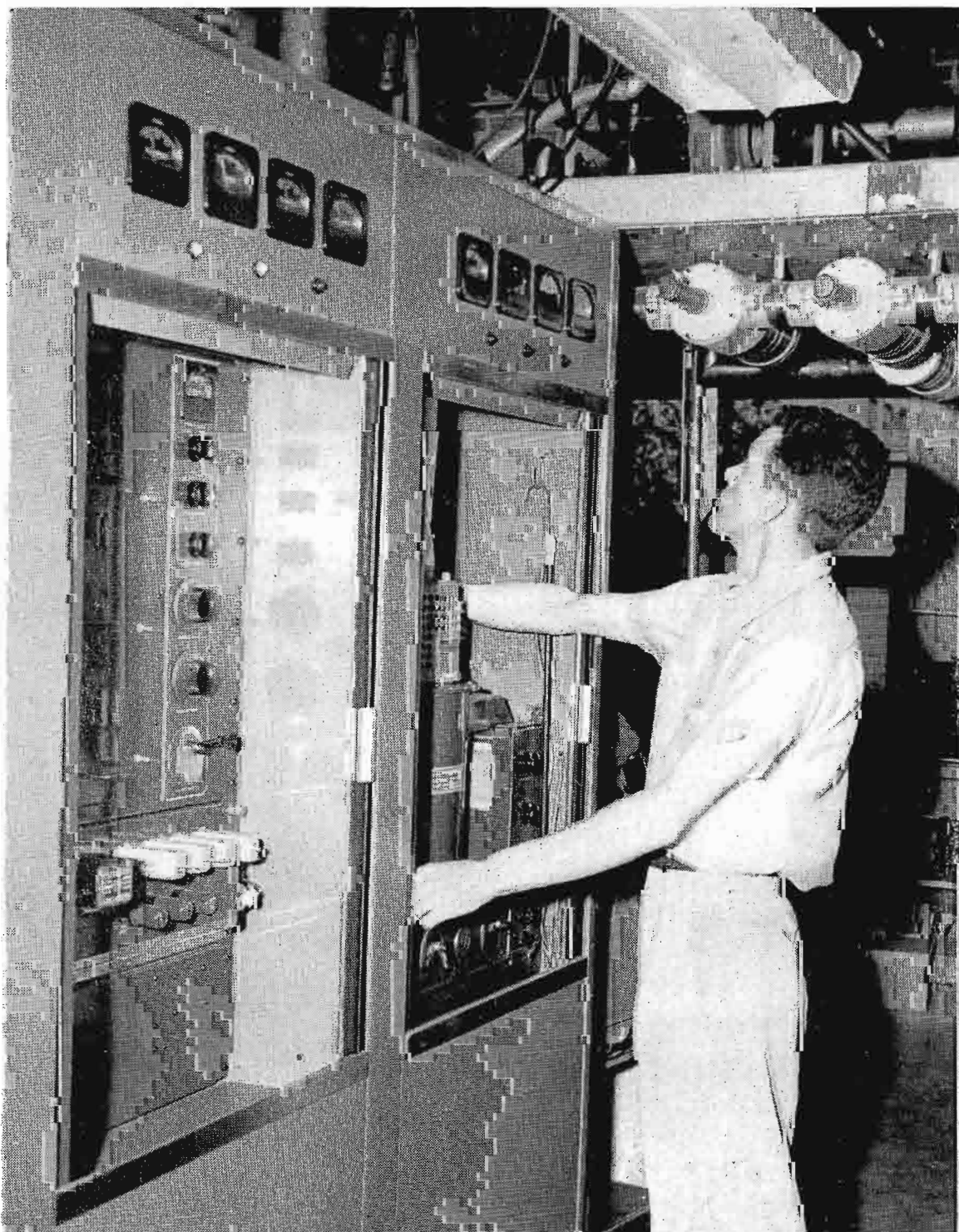
FIG. 12. Hugh Mulhollam, Transmitter Technician, is shown tuning the Visual Exciter Section of the TT-10AH, RCA 10 kw VHF Transmitter.
