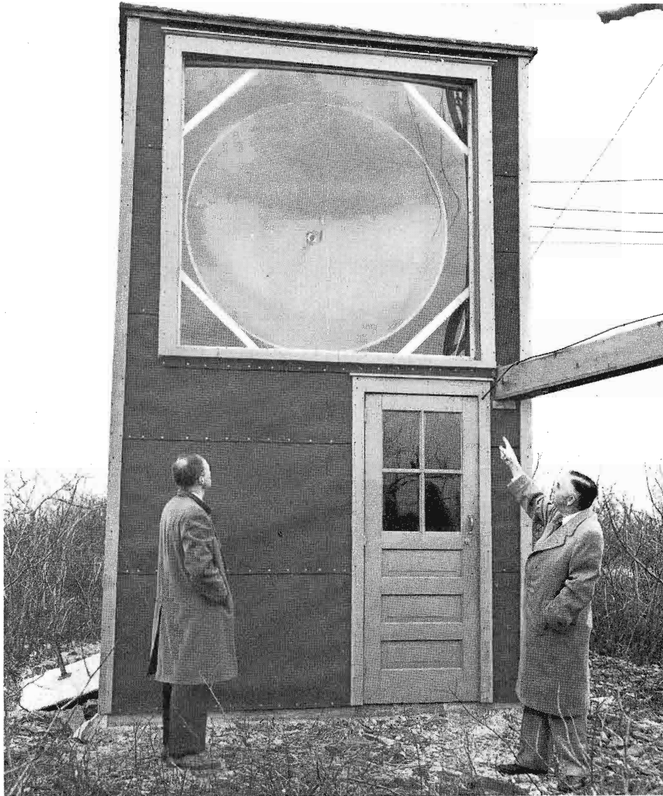
Closeup of relay transmitter housing at Pimple Hill. Network service is relayed from this point, 70 miles air distance from New York. Pimple Hill station is the main inter-city relay connection. ▶
